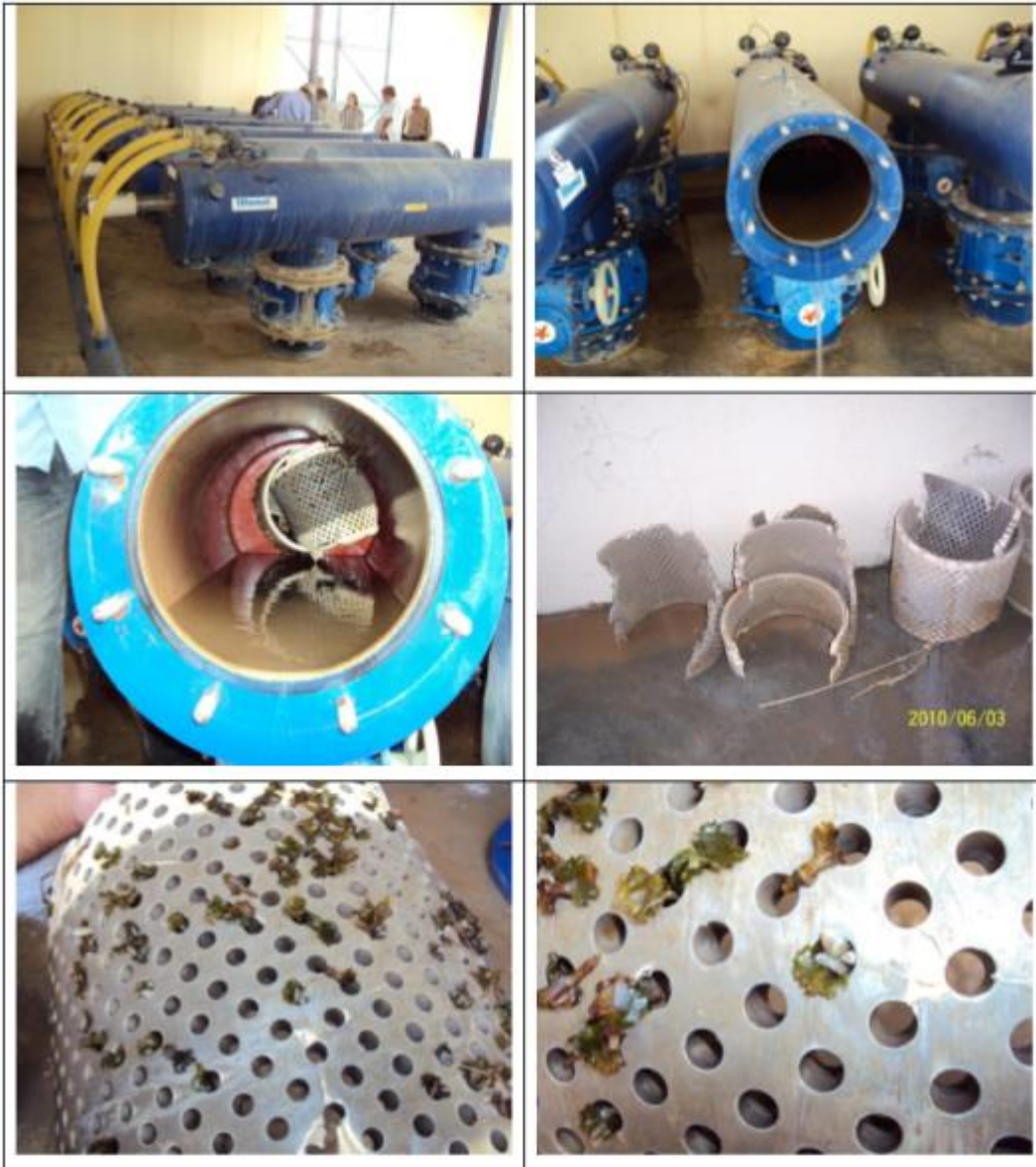
Figure 13 .Urfa Bozova Irrigation Pump Station's Filters in 2010 (21)
