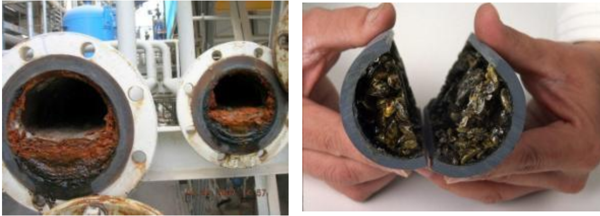
Figure 16. Zebra Mussel accumulation in the pipes.
