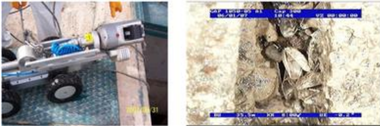
Figure 17. Robotic Camera and Zebra Mussels accumulation into the connection part of the pressured CTP type pipe (21).
