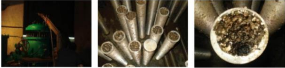
ATATÜRK Dam HEPP Cooling system
