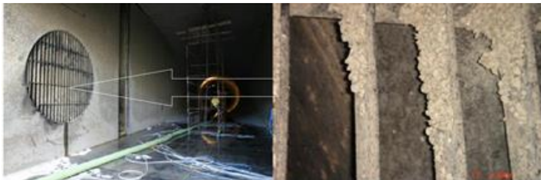
Figure 14. Zebra Mussel Accumulation on the Urfa Tunnel Raw Drinking Water Intake (21)
